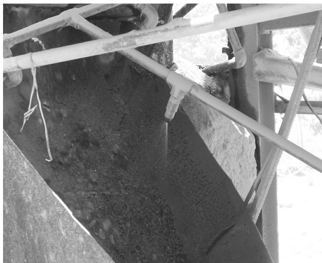
Spray nozzles strategically placed in the stone crushing unit help to significantly decrease the generation of respirable silica dust.
