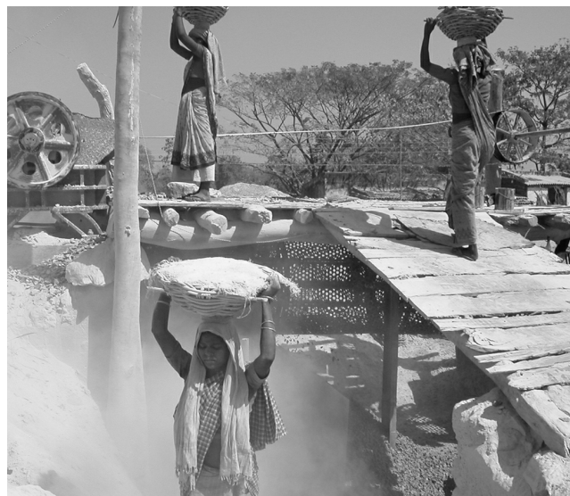
Workers manually loading the crusher unit and hauling off fine materials accumulating under the rotary screen while continuously exposed to airborne silica.
